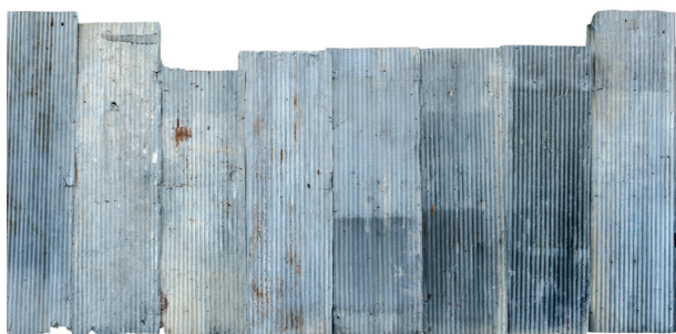
Fig 10.7 Damaged iron sheets
